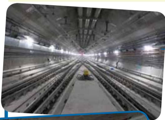
設有消防員旁邊的鐵路隧道。 Fireman's walkway at the railway tunnel.
