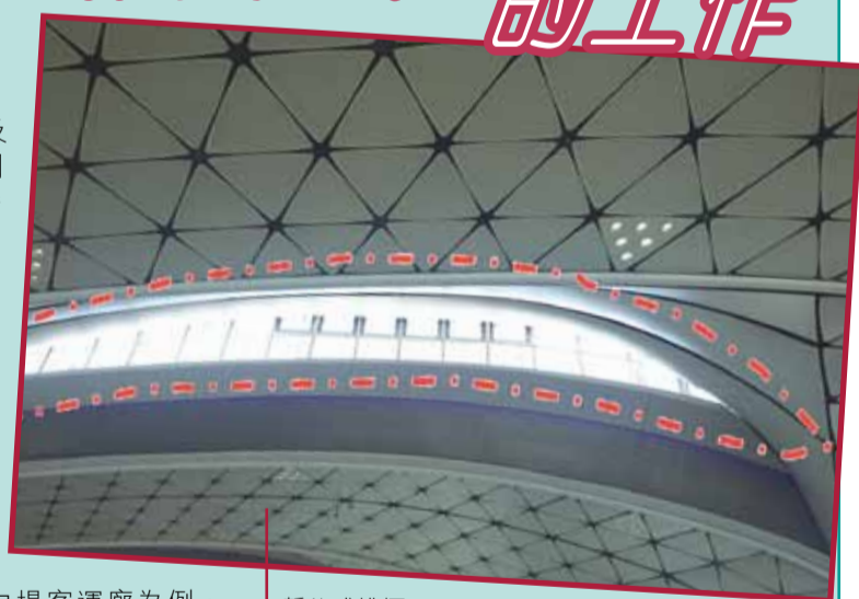
靜態式排煙口。 Smoke vent of static smoke extraction system.
