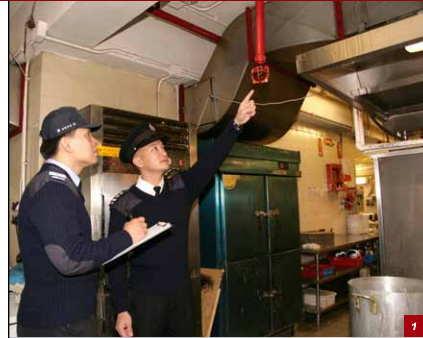
1 消防人员巡查食肆的消防设备 Fire personnel inspect the FSI in a restaurant
