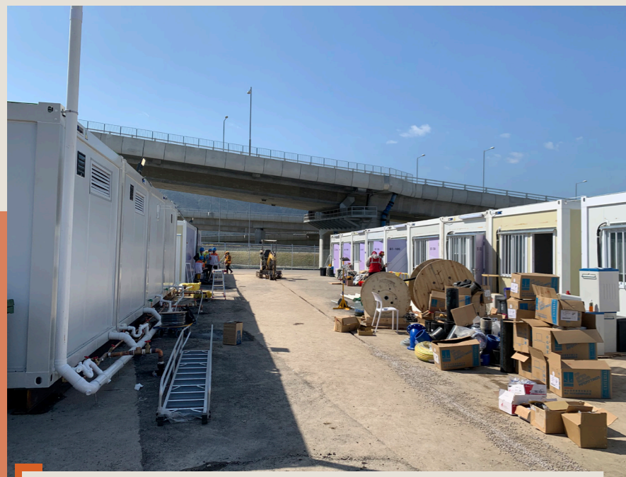
消防處籌組「抗疫設施驗收小隊」，加快驗收社區隔離設施的消防裝置及設備。 The Fire Services Department forms Anti-epidemic Facilities Acceptance Inspection Teams in order to accelerate FSI acceptance inspections for community isolation facilities.
