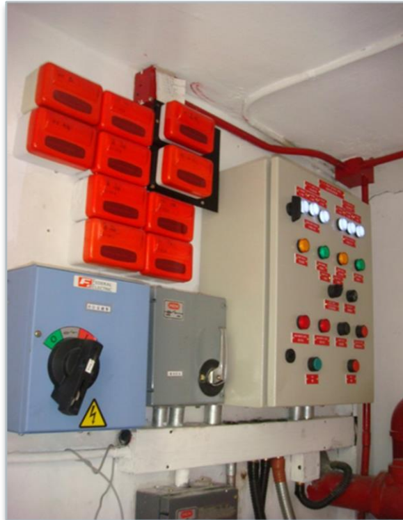
Fire Pump power supply switch (electrically fail test)
