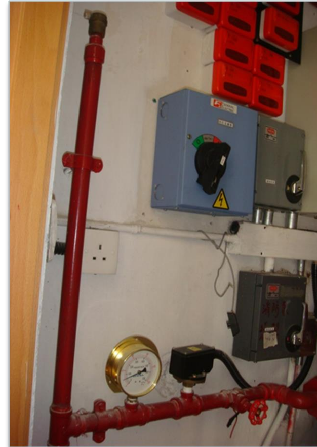
Fire Pump pressure switch (mechanically fail test)
