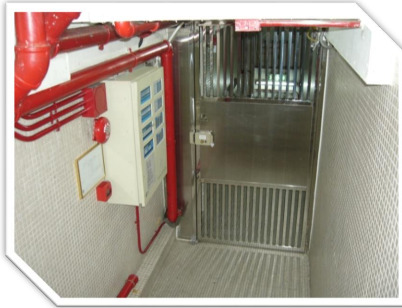
Fire alarm panel
