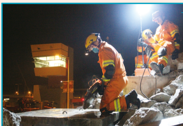
拯救人員利用工具切割混凝土。 Team members cutting a concrete block.
