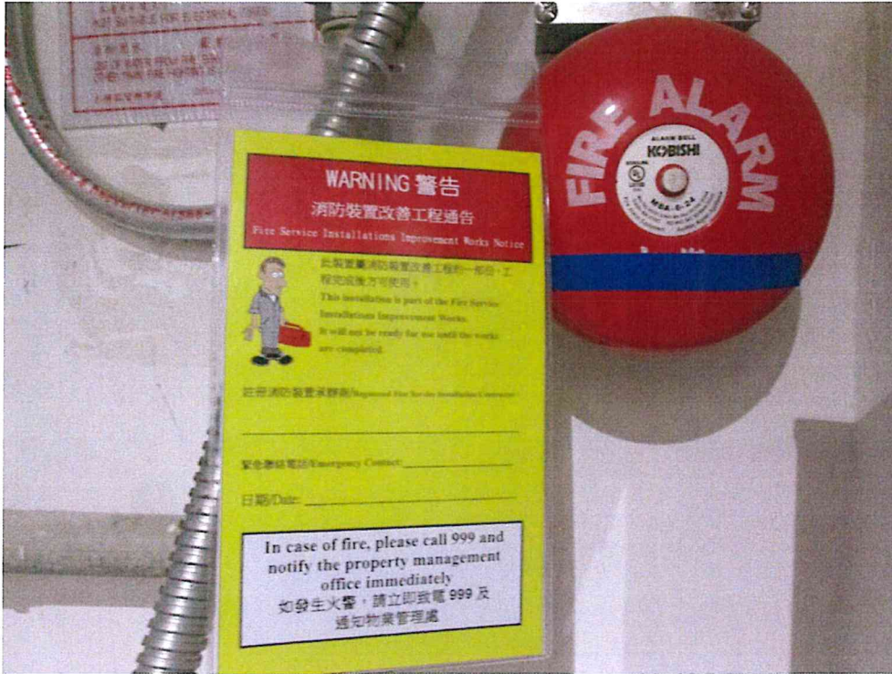
Fire Alarm Bell
