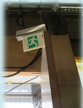
Incomplete Exit Sign
