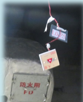
Incomplete Fire Alarm
