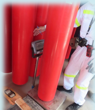
CO2 Cylinder found under-weighted
