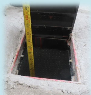
Spindle of Underground Hydrant Valve not within the requirement
