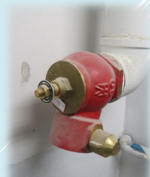
Incomplete FS Outlet
