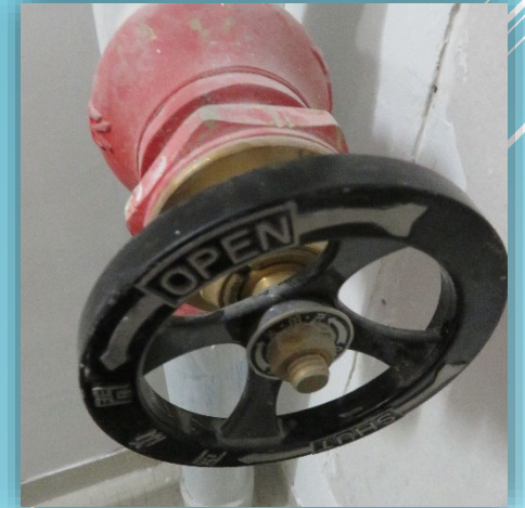
Hand-wheel's operation ineffective
