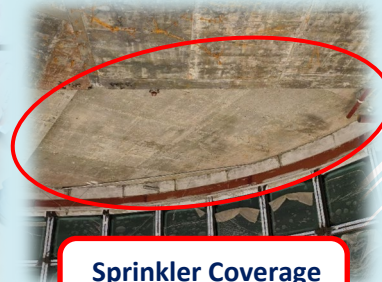
Sprinkler Coverage found inadequate
