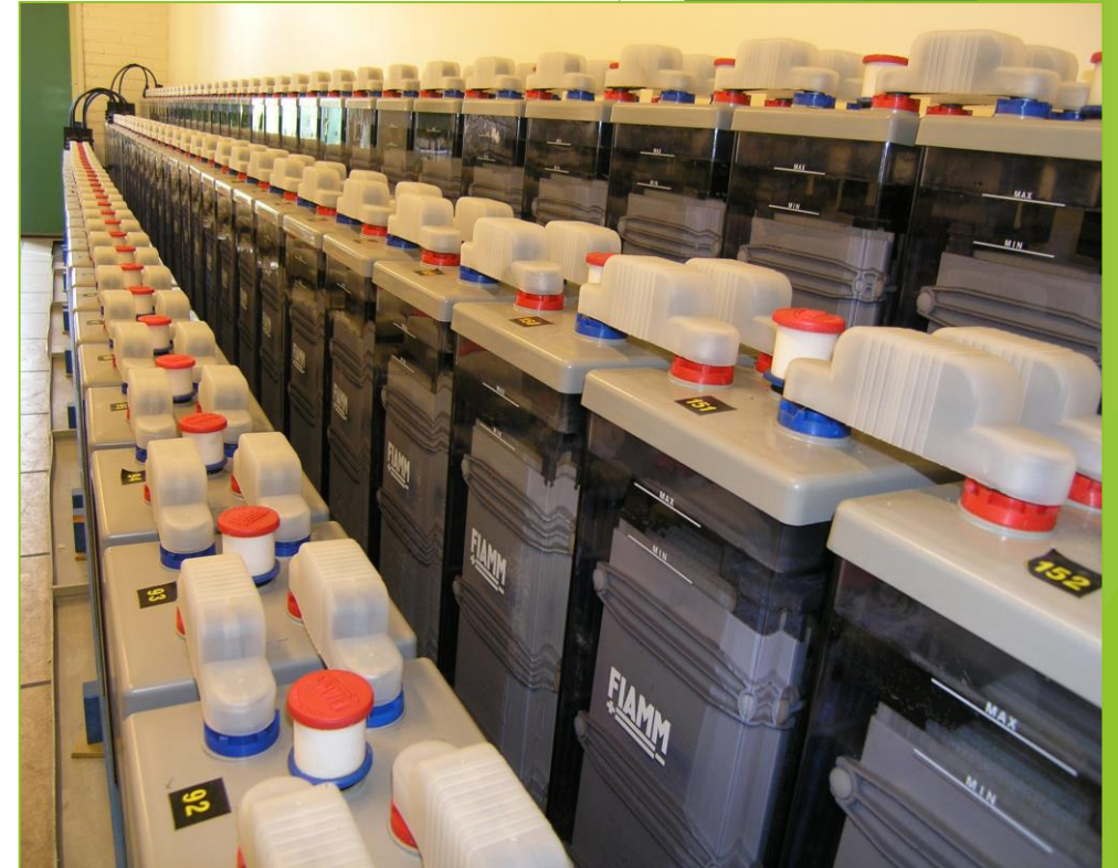
Image from https://servicepoolen.com/en/news/ventilation-in-battery-room
