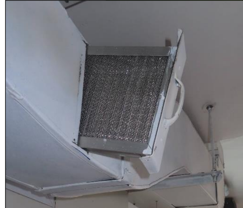
Intake air filter
