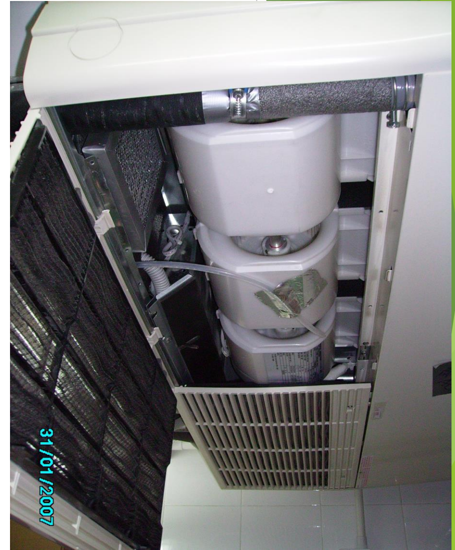
Example 3 PVC blower fan casing and nylon filter inside return air plenum of A/C unit were not accepted.
