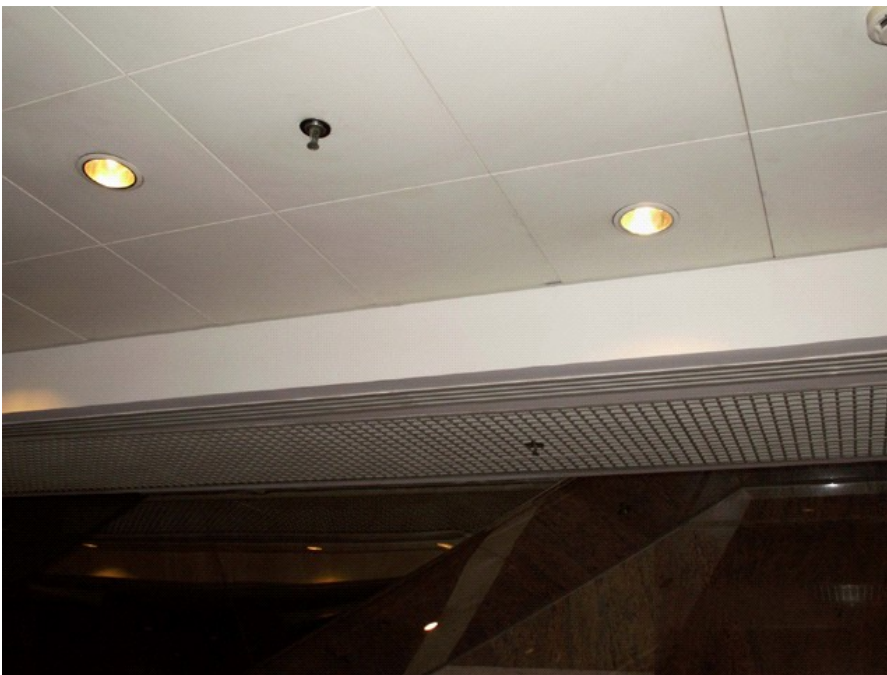
Sprinkler head clear of any obstruction
