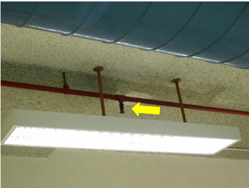
Obstruction to sprinkler head
