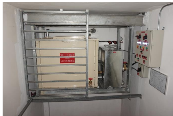
Supply Tank of 500-litre installed inside Roof-floor Staircase
